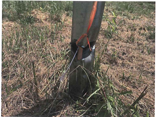
The casing associated with MW-2D has been damaged and the PVC riser has been clean cut. The riser is now approximately 1 foot above grade. Replacement of the casing and repair of the riser is necessary.
